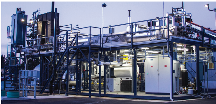
Figure 2. The Commercial Unit being tested in Washington, USA, prior to being delivered to and assembled in Dakar.
